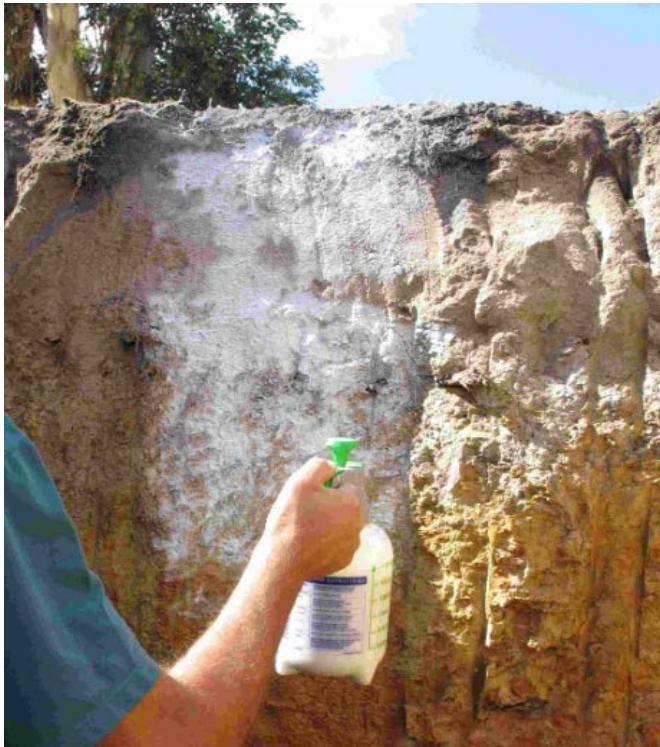
Figure 2 First coat of latex is a diluted spray of about 50 per cent latex and 50 per cent water
